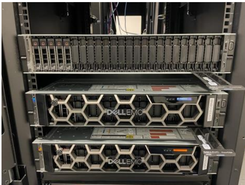
Figure 5. Testing Hardware: 3 x DELL Power Edge R750 S
